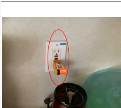
GFCI not working
