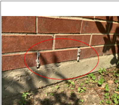
Improperly caulked weep holes
