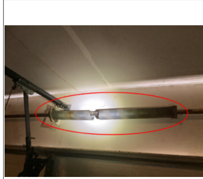
Garage door spring is broken. I recommend repair by a specialist.
