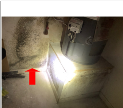
Organic mold-like substance found on garage wall near hot water heater. It's possible this could be from previous plumbing pipe damage behind wall or a current leak situation. I recommend evaluation by a specialist.
