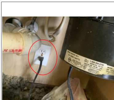
Waste disposal not GFCI protected
