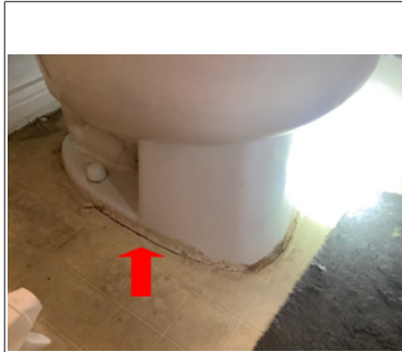
Commode base loose and needs proper caulking/sealant.
