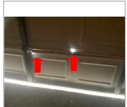
Steel garage door panel has holes in it. In most instances the holes cannot be repaired, however the entire panel would have to be replaced. 2 panels show damage.
