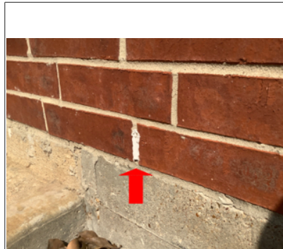
Improperly caulked weep hole
